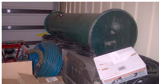
The unused ultraviolet disinfection system (EPA OIG photo)
